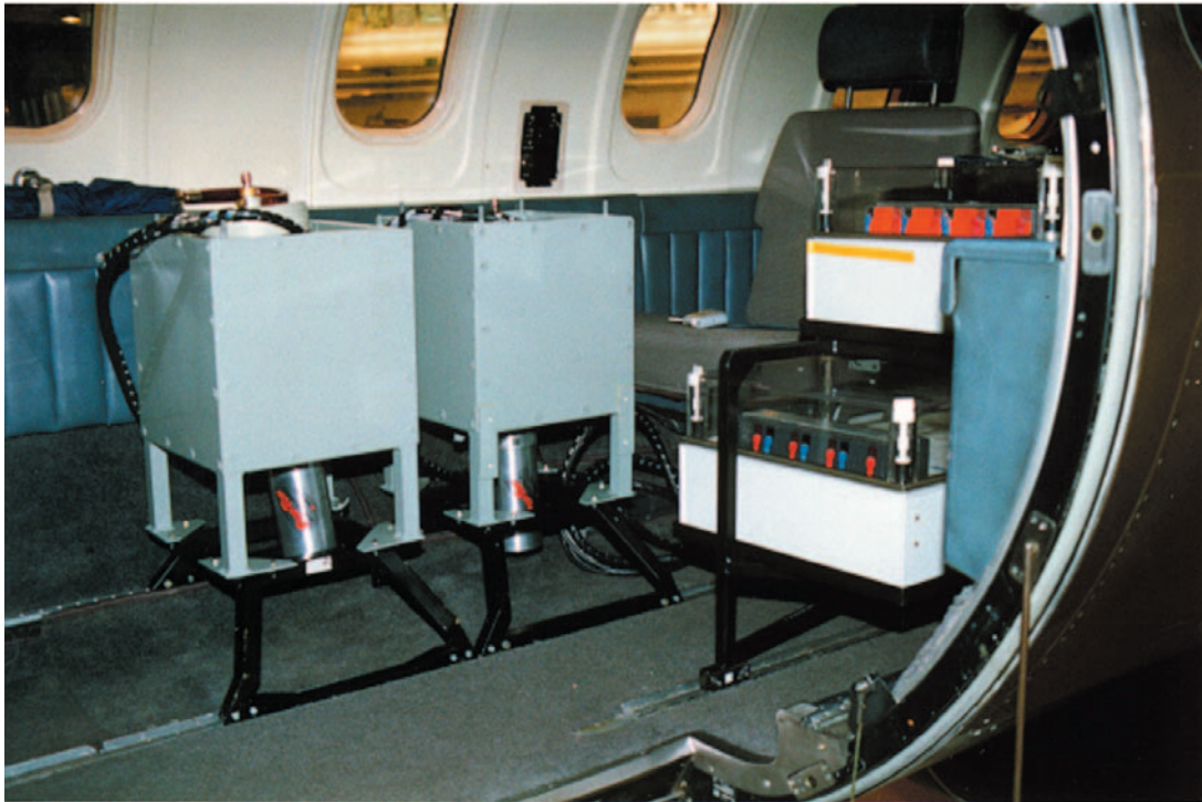
Figure A1-3. An example of typical equipment installation accepted for continuous use in Finland. In this case two HPGe-detectors were being installed. The first HPGe detector was not completely in place.
