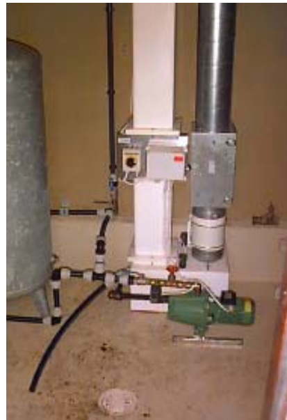
Figure 5. The Gagnef waterworks, where a Czech packed tower aerator is applied for radon removal. A pressure tank is located on the left, the inlet air duct (in the right) is equipped with a channel blower, which helps the incoming air to flow downwards through the air filter (inside the upper part of the duct) and then upwards in the narrow packed column located in the middle.
