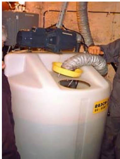
Figure 8. In the Mons Samf. waterworks in Siljansnäs radon is removed with a RADON-X magnum aerator equipped a plastic aeration tank. The water level is easily visible due the dark colour on the inner surface of the tank. The colour is probably caused by the precipitated manganese hydroxide. No manganese removal is however needed due to its low content in water. The radon rich air is exhausted to the outdoor air through the ventilation duct, which has just been opened in the figure.
