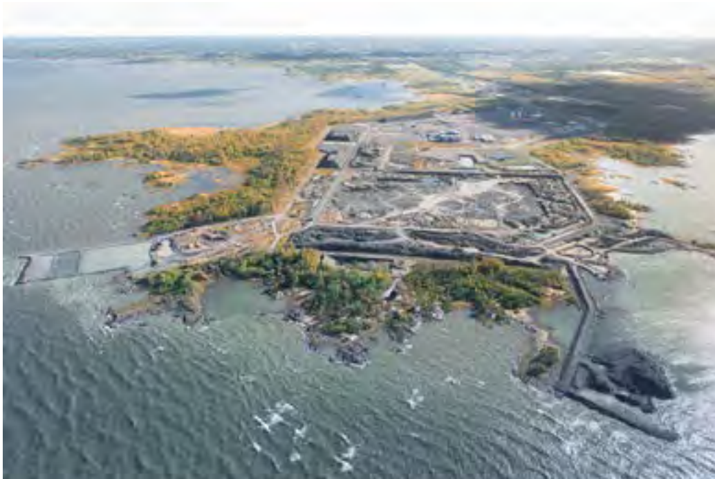
FIGURE 29. Hanhikivi site in Pyhäjoki under site preparation and additional site surveys during the Autumn 2018. Source Fennovoima.
