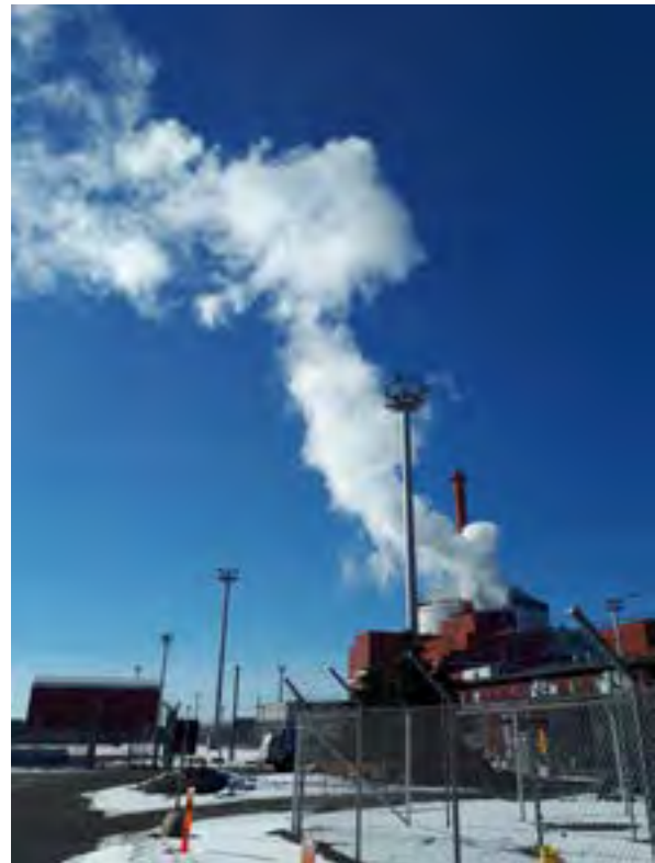
FIGURE 26. Commissioning tests of main steam relief trains at Olkiluoto 3. Source: STUK.
