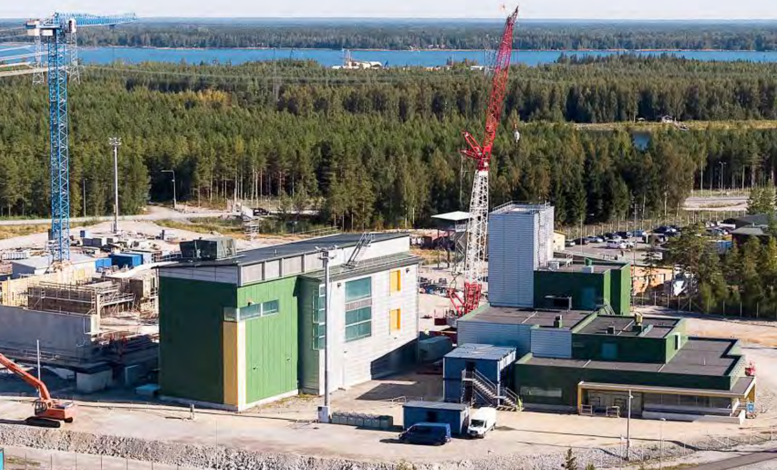
PICTURE 1: Encapsulation plant of the Onkalo under construction in 2020. Outer structure of the spent fuel disposal canister is made of 5 cm thick copper, that mainly acts as a corrosion barrier. Pictures: Posiva.
