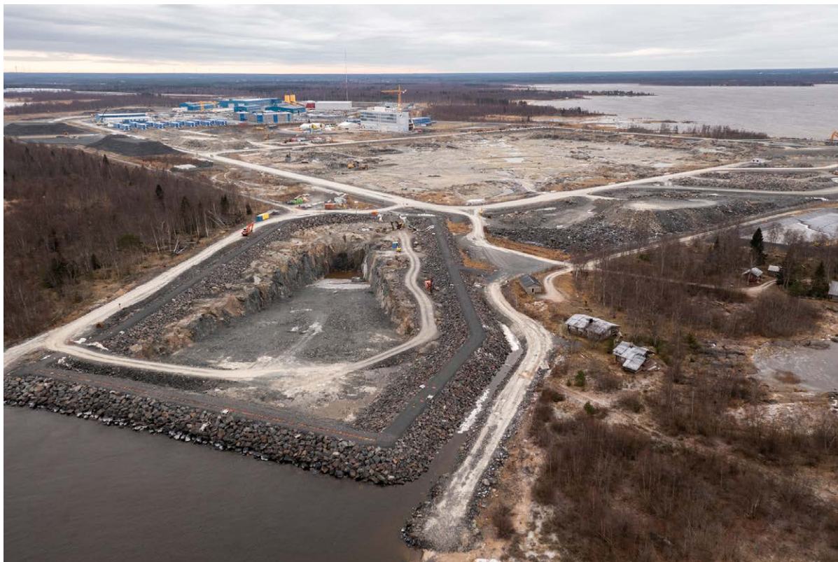
FIGURE 26. Hanhikivi site in Pyhäjoki: At front cooling water outlet channel with temporary dam and on the background NPP plant pit excavation down to –2m (FH1 November 2021). Source: Fennovoima.
