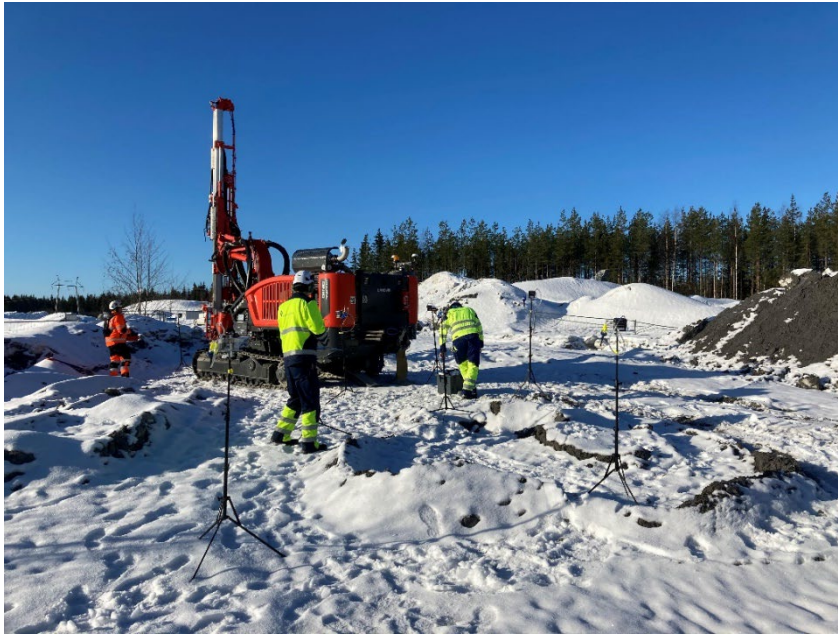
Figure 4. Measuring quartz dust emissions of a drilling rig in a test field.
